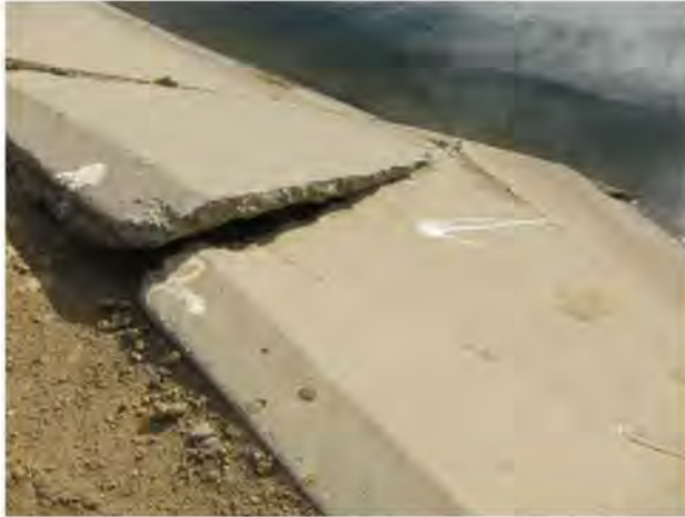
(Cracks and buckle along Delta Mendota Canal. Photo By Amy Quinton)
